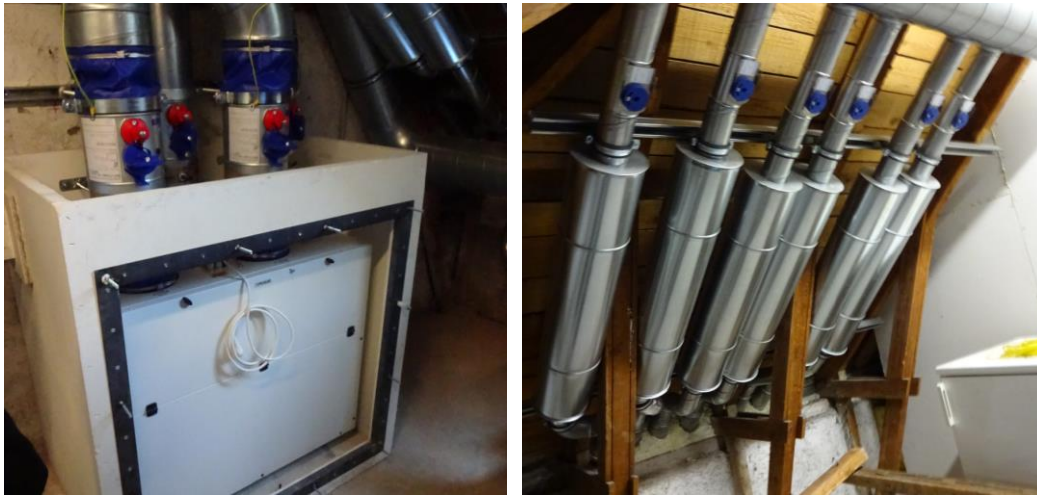
Figure 2: Left: Central unit with fire protected housing and fire dampers at the top. The fire protected maintenance cover at the front is not mounted in the picture. Right: Supply air ducts in attic with flow regulation dampers, silencers and penetration to the outside of the exterior wall.
