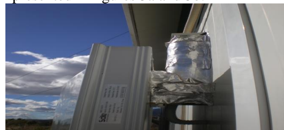
Figure 5b: Measurements point at the modified air outlet
