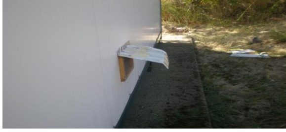
Figure 6a: Ventilation inlet
