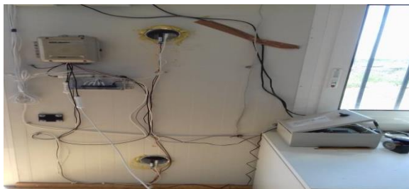
Figure 4a: Measurements points at the air duct
