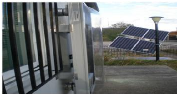
Figure 3: Installed solar air collector
