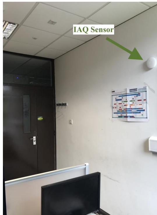
Figure 1. A IEQ sensor mounted on the wall in an office.
